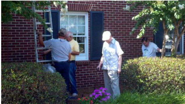
Members assist with the ground work. Here, Mac Cullom, K4AVR, is preparing a balun.
